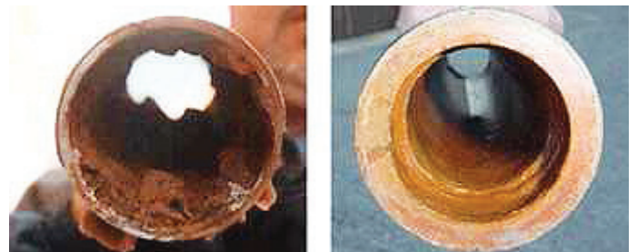
removal of biofilm
